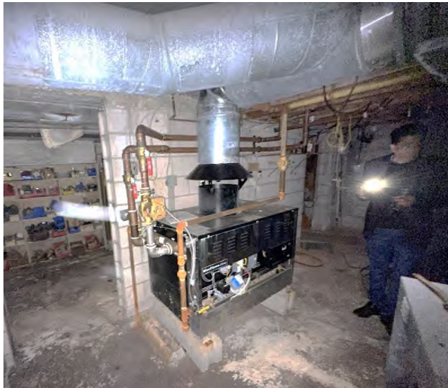
Picture on Left was taken Aug-29-2025 of the Boiler/Furnace located in the basement
