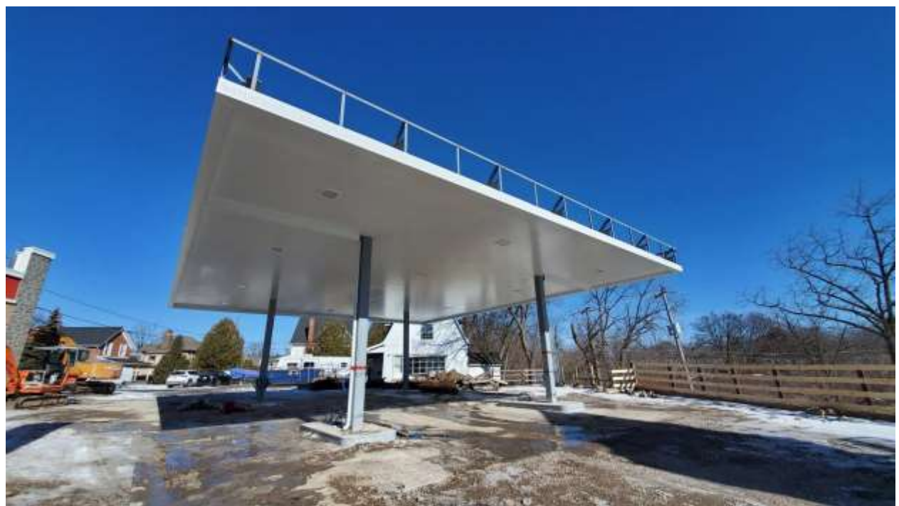
Future Fuelling Facility
