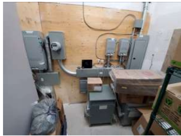
Main Electrical Service
